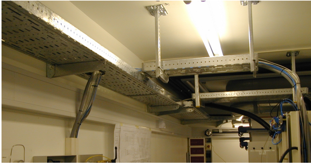
Figure 2-6: Overhead cable raceway
